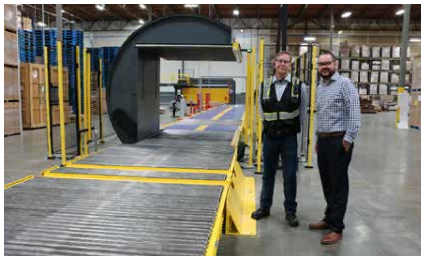
Bill Sterkel, Maintenance Manager at Bay Cities, left, and Mark McGinnis of Systec Conveyors next to the new load inverter and conveyor line.
